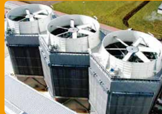
Mechanical Draft Air Cooled Condenser (ACC HEXACOOL)
