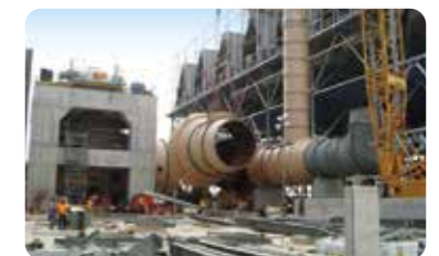
Goreway Canada 880MW Combined Cycle Power Plant
